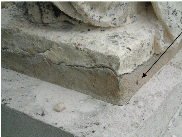
4. The failed cement repair to the base of Faith, before removal.
