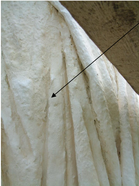
12. Detail of a section of Faith's drapery after dentistry mortar repairs and 2 coats of lime wash.
