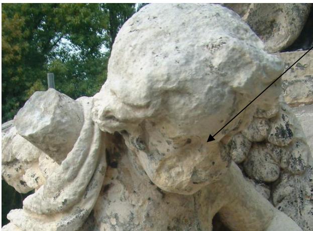
13. The deteriorated carved detail on the head of the left side cherub before mortar repairs were carried out.
