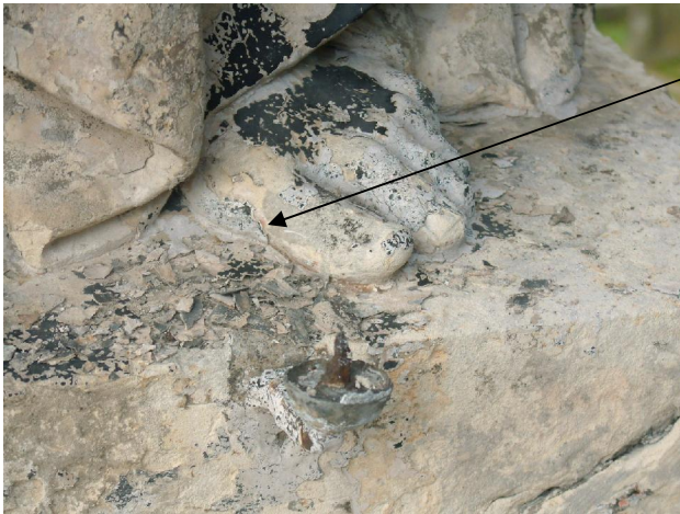
1. The loose paint layers on the stone work.
