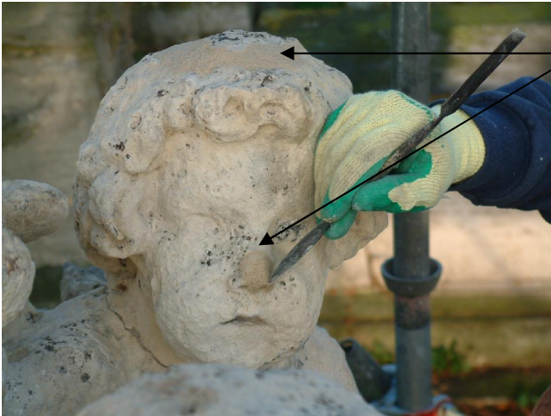
15. Mortar repairs being carried out on the deteriorated carved detail of the right side cherub.
